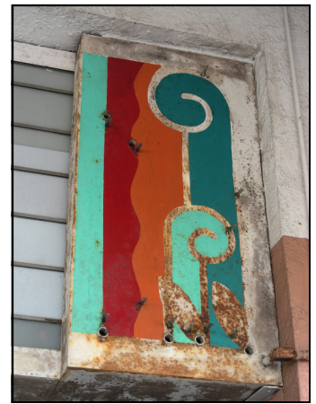
Rusted marquee ends prior to restoration
